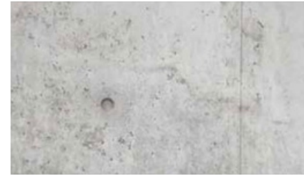
New concrete with slight blemishes
