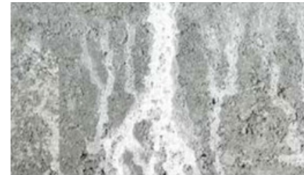
New concrete with severe blemishes
